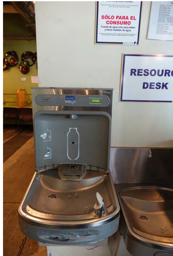
Water bottle filling station in the main lobby waiting area. Austin Research Center for Homelessness. Architecture by LZT Architects and Herman Thun.
